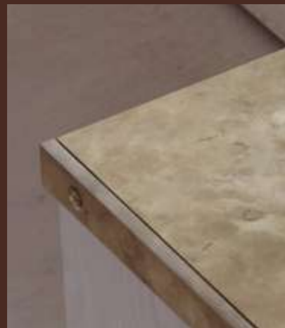
Brass sheeting and angles – unsealed
